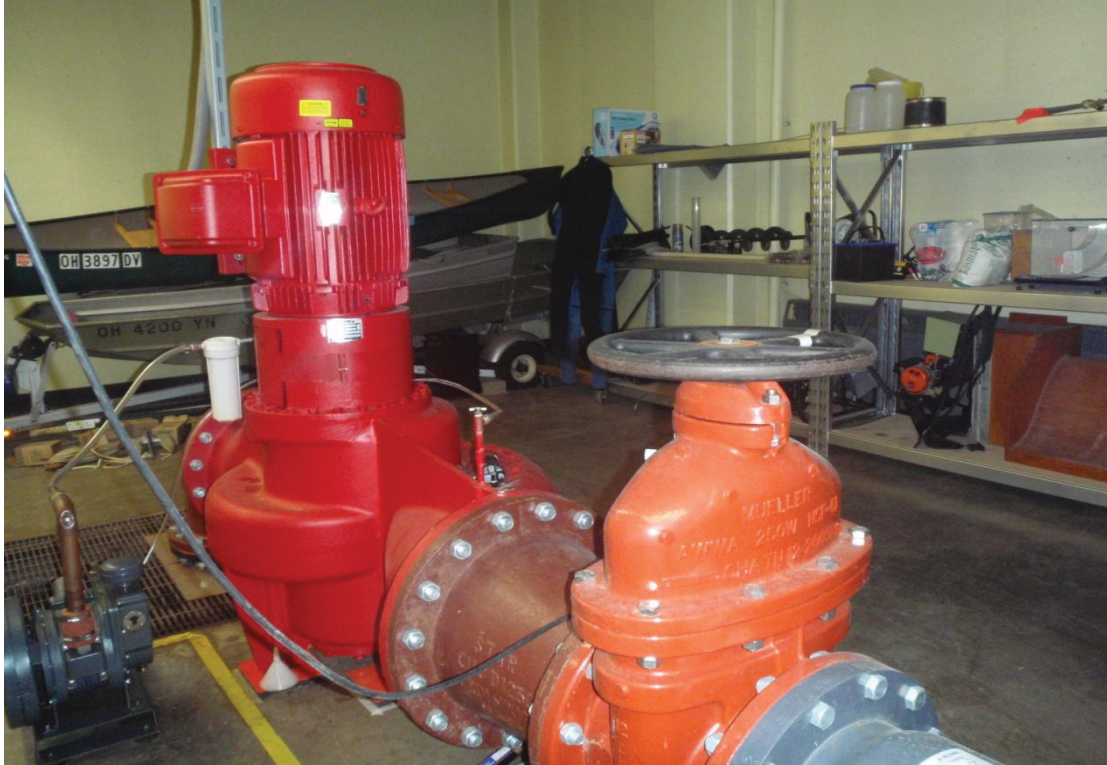
Picture showing Pump and valve
