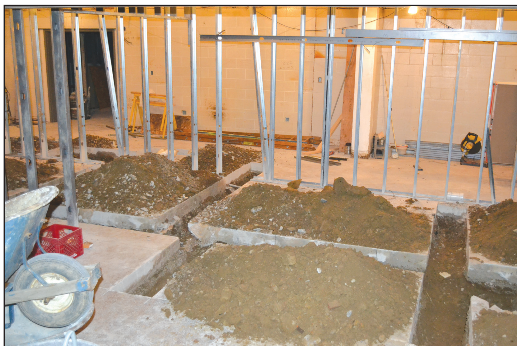
The date that Wendy's was expected to open in Kilcawley Center came and went on Monday as construction continues. Photo by Kacy Standohar/The Jambar.
