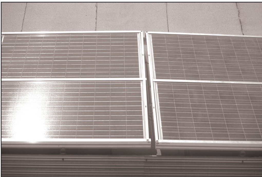
Solar panels stretching across 41,000 square feet of Moser Hall's roof provide electricity for the building and serve as a teaching tool for engineering students at YSU. Photo by Christina Mullen/The Jambar.
