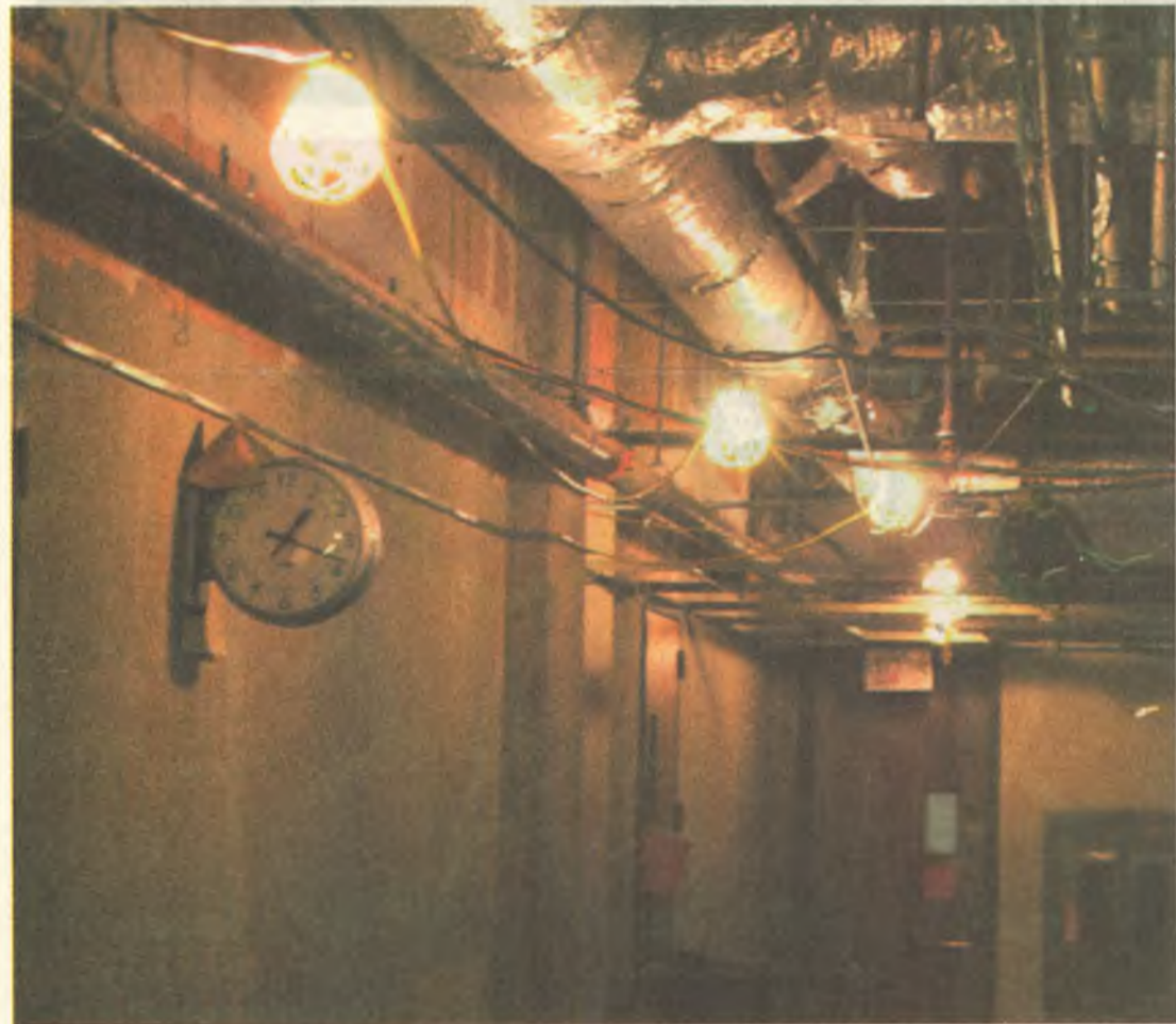
Lights line the ceiling of the basement of DeBartolo Hall during renovations taking place this summer. DeBartolo Hall will undergo two phases of renovations, costing $1.9 million. Photos by Matthew Roth/The Jambar.
