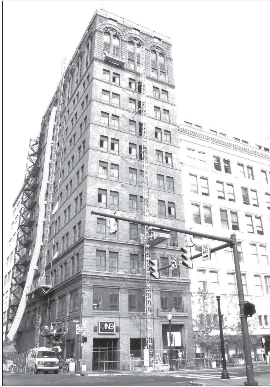
Wick Tower, on the northeast corner of W Federal and N Phelps Streets downtown, is currently being renovated. The building will contain 50 apartments and have commercial space available on the ground floor.
