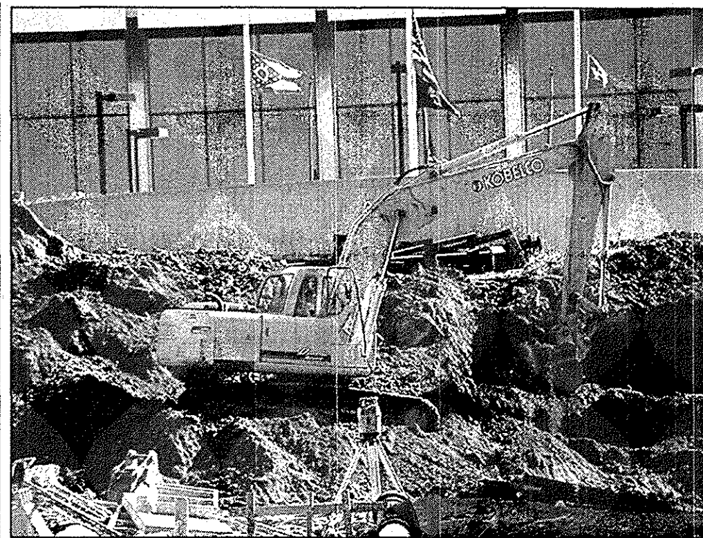
► Construction crews work to catch up to their project deadline after persistent rains impeded progress in building the new Andrews Student Recreation and Wellness Center. The Wellness Center is a part of YSU's West Campus Gateway project and is expected to open in August of 2005.
