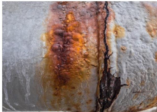
Figure 1.9. Stress corrosion cracking [103]
