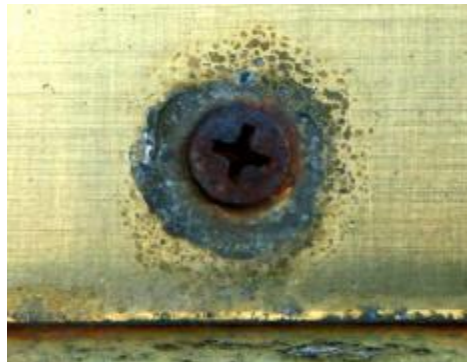
Figure 1.7. Galvanic corrosion of two dissimilar metal [111].
