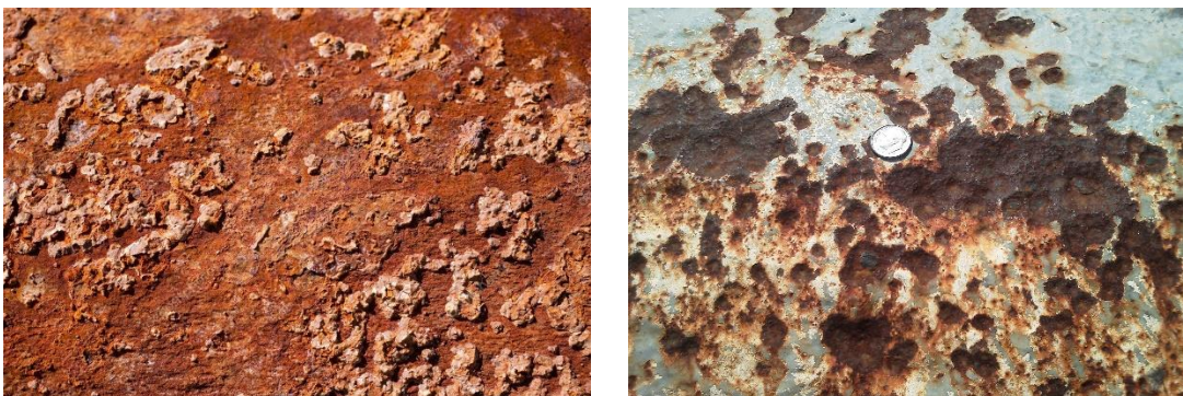
Figure 1.1. Example of corroded surfaces [103]
