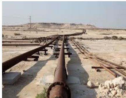
Figure 2.2. External corrosion of pipeline [121].
