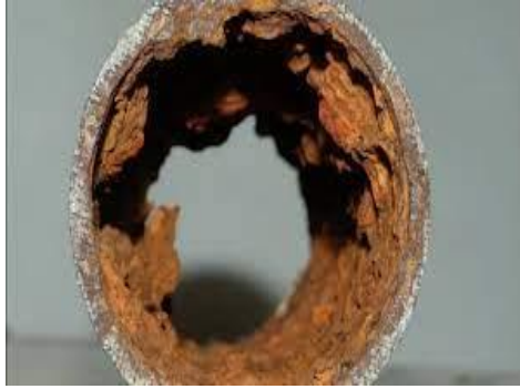
Figure 2.1. Internal corrosion of pipeline [120].
