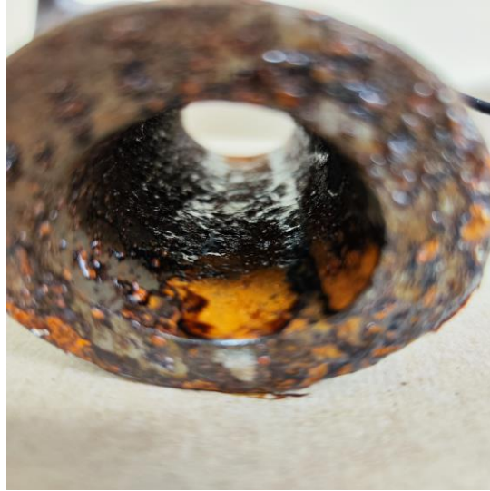
Figure 4.31. showing a closer look at the internal corrosion of the metal pipe after the 8 weeks period.
