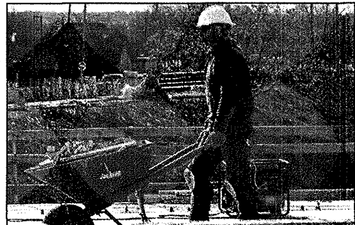
A worker carries a load of wood across the Fifth Avenue bridge, which crosses Route 422, on Monday. The bridge is one of six under renovation in a $7.5 million ODOT project.
