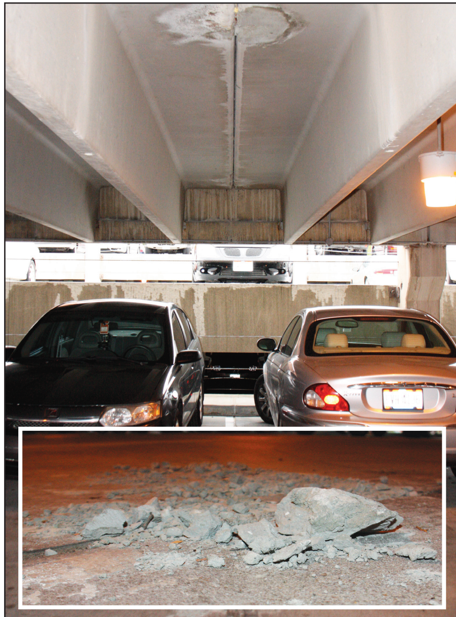
A chunk of concrete (pictured above) fell from the M-2 parking deck on Friday. This damage comes after extensive renovations over the summer. Photo by Dustin Livesay/The Jambar.
