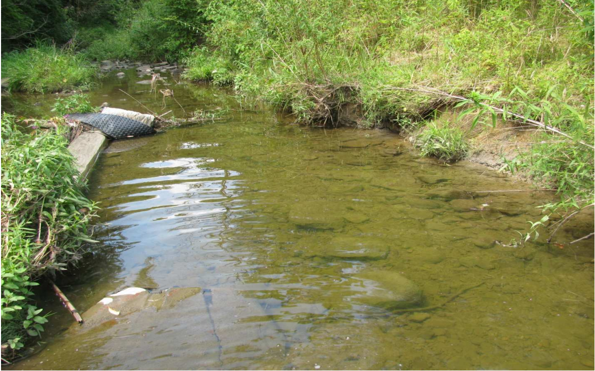
Figure 4.16 Debris jams on restored reach of Indian Run (July 2010).
