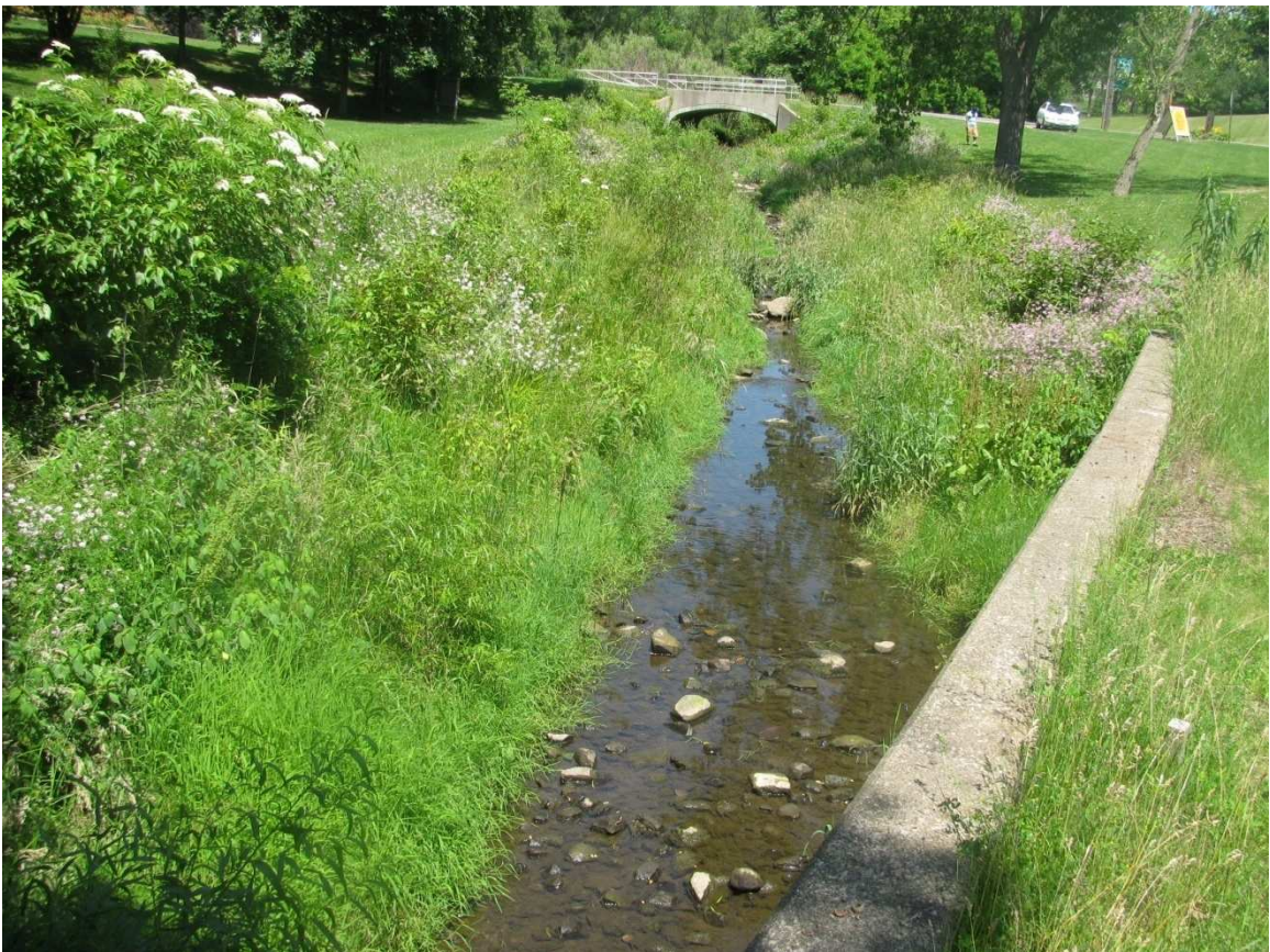
Figure 4.4 Debris and channel blockages in restored channel reach looking upstream at Austintown park site (June 2010).
