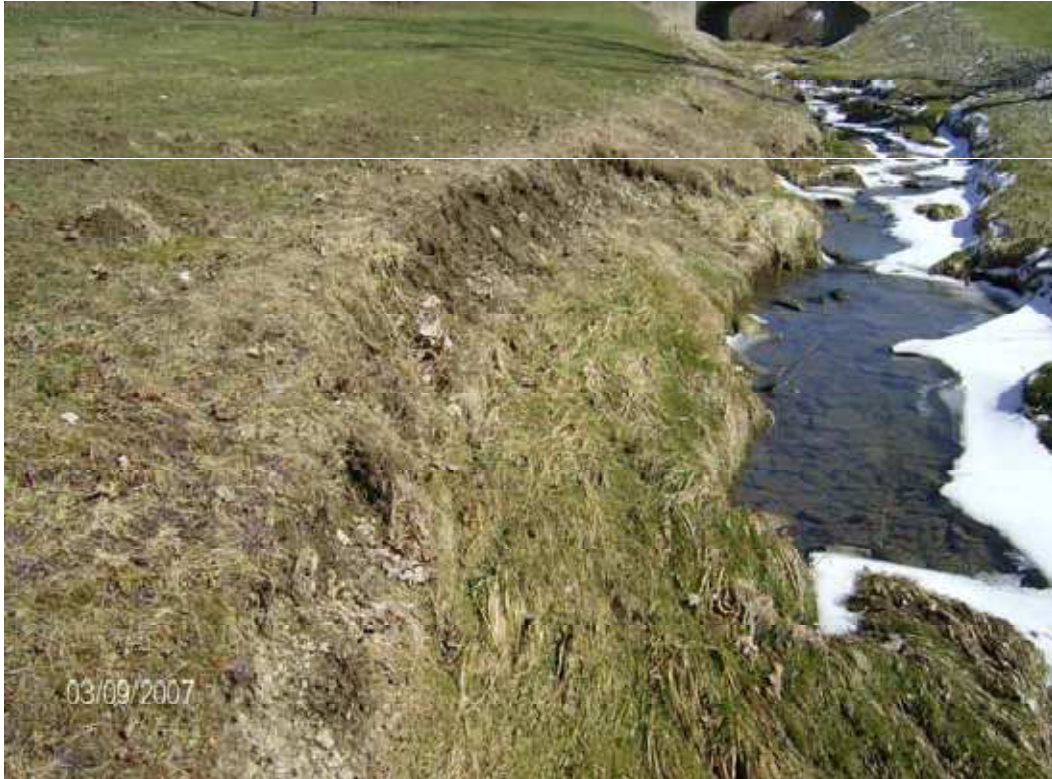
Figure 2.11 Sliding and eroding bank on the north bank of the Austintown Park stream (WPI 2007).
