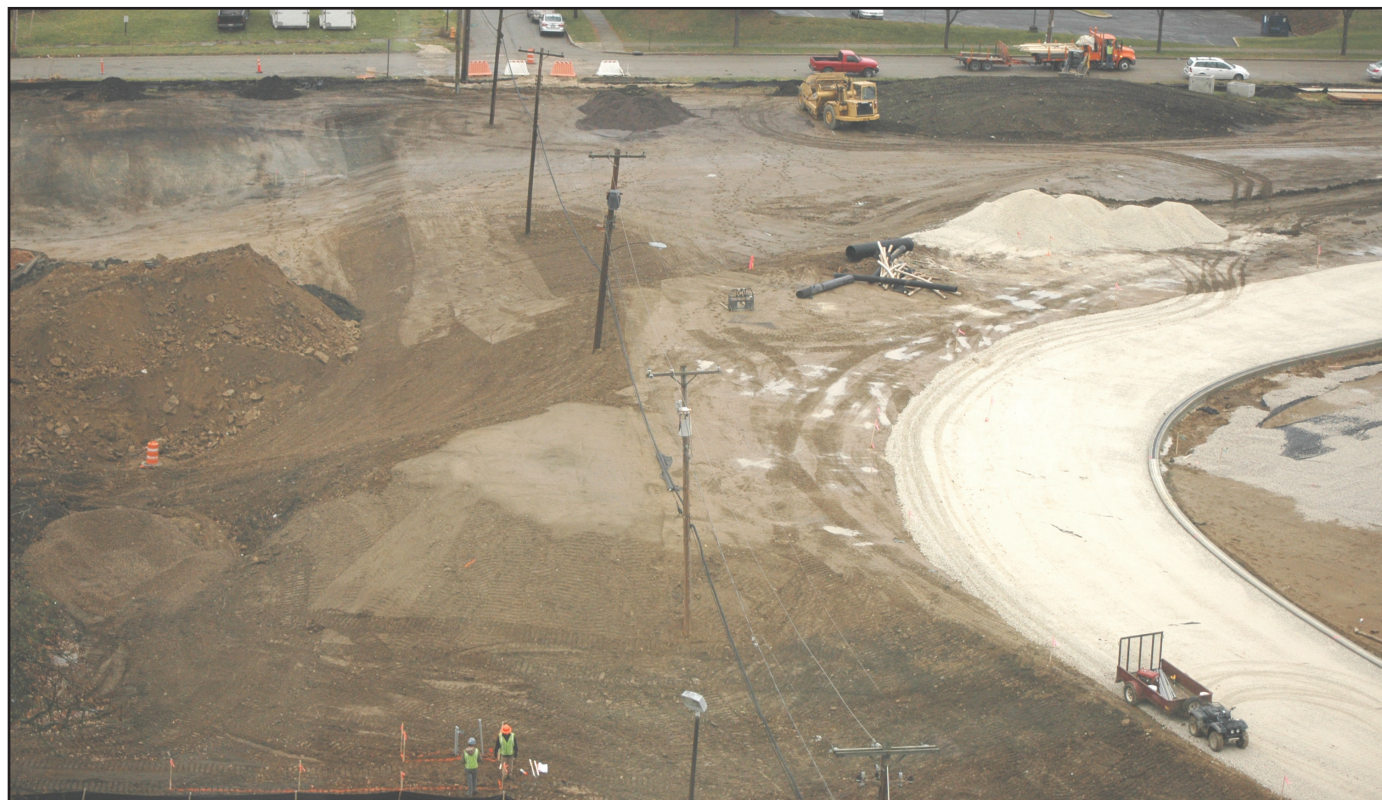
Construction continues on the new athletic facilities. To the left is the area being prepped for the softball field, and to the right is the soccer field and track. Photo by Cory Bartek/The Jambar.
