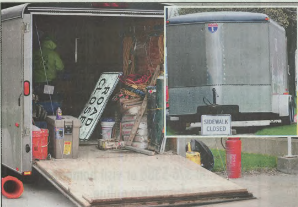
Renovations of the M-2 parking deck at the corner of Lincoln and Fifth avenues began Monday, closing the deck to students. Parking opened to YSU students at the Covelli Centre in downtown Youngstown. Renovations are expected to last throughout the summer, and the deck is predicted to reopen for the fall semester. Photos by Chelsea Telega/The Jambar.
