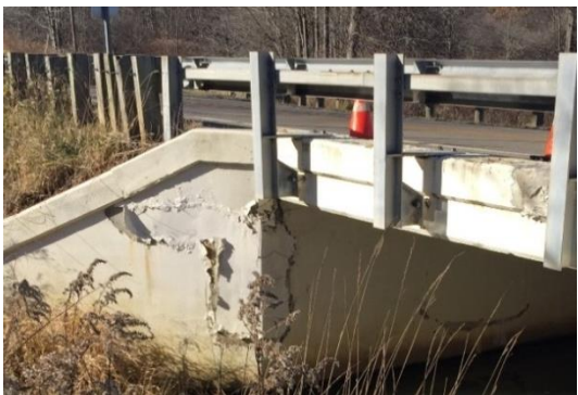
a) Cracks on the wing wall
