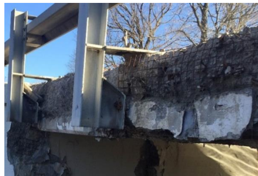
b) Deterioration of curb surface
