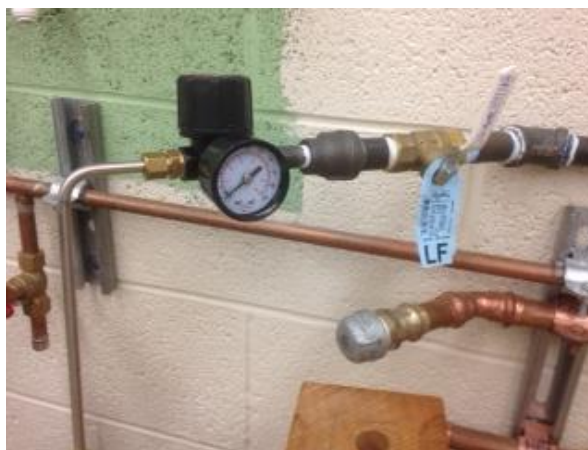
Figure 14: Air inlet with pressure regulator.
