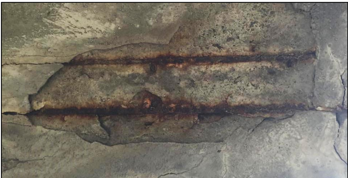
Figure 1-3: Close-up picture showing corroded reinforcement.
