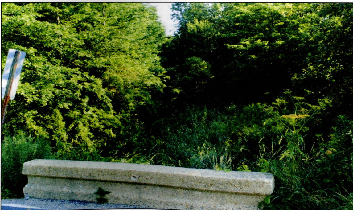
Figure A.2 Candidate Parcel mn33, Looking North at culvert from South boundary
