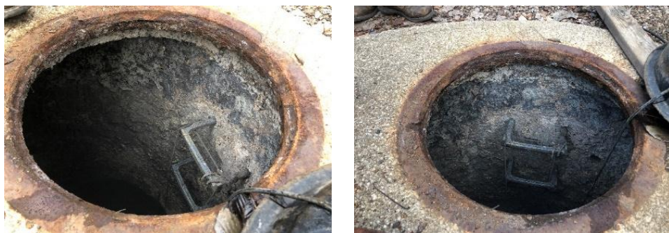
Figure 3-4, Severe deterioration of wet well at Meadowood Circle location , Poland, Ohio (pictures by Mostafa Nasr)
