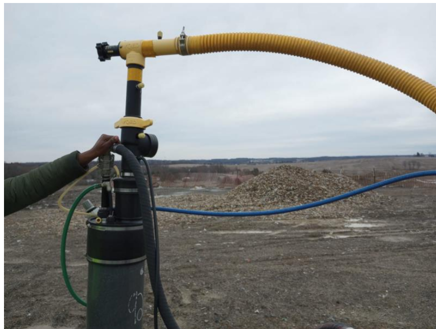
Figure 3.29: Wellhead for landfill gas at the Mahoning Landfill.
