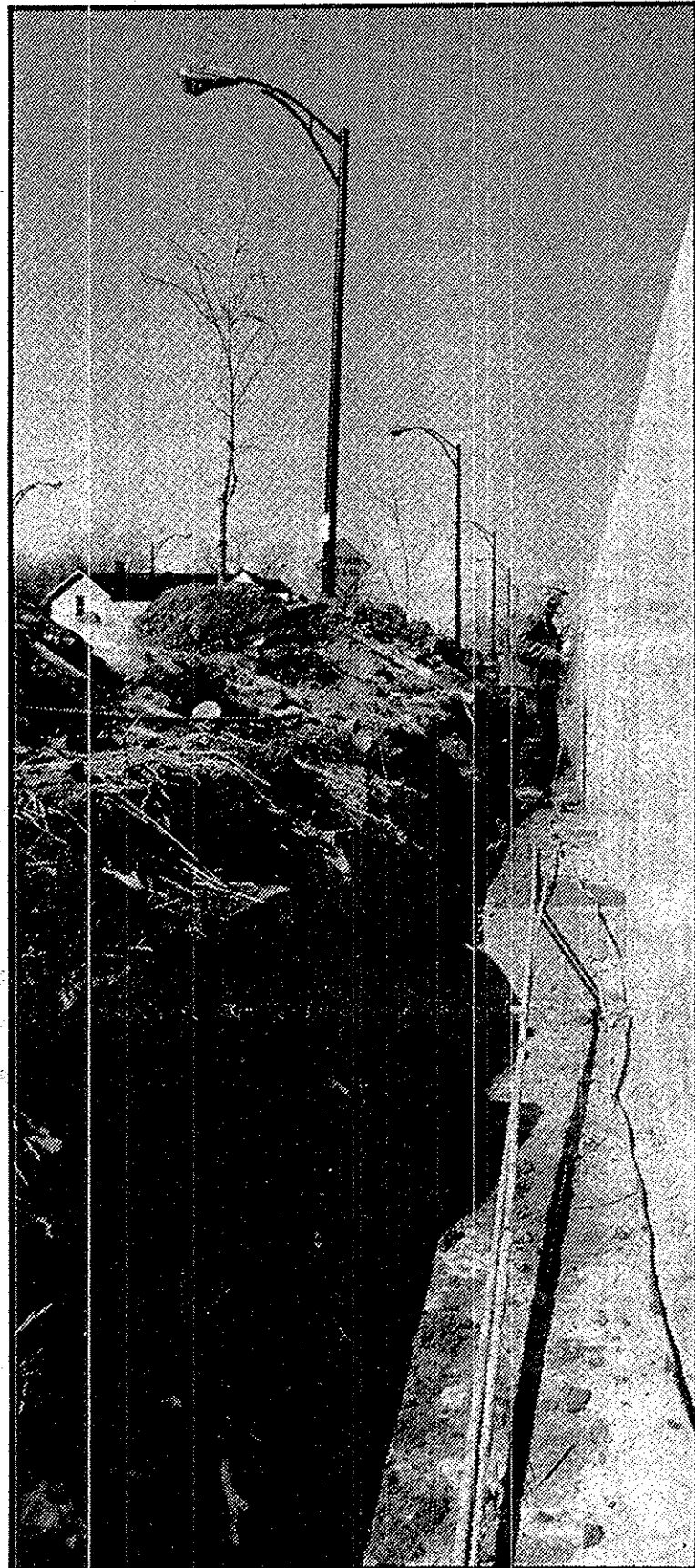
A worker sands a concrete retaining wall that, when final touches are completed in two months, will span the length of the sidewalk between the Madison Avenue Expressway and Spring Street on Fifth Avenue. The wall will support earth to be landscaped up to a new driveway slated to stretch along the front of the All-Sports Complex. (Photo by John Celidonio)
