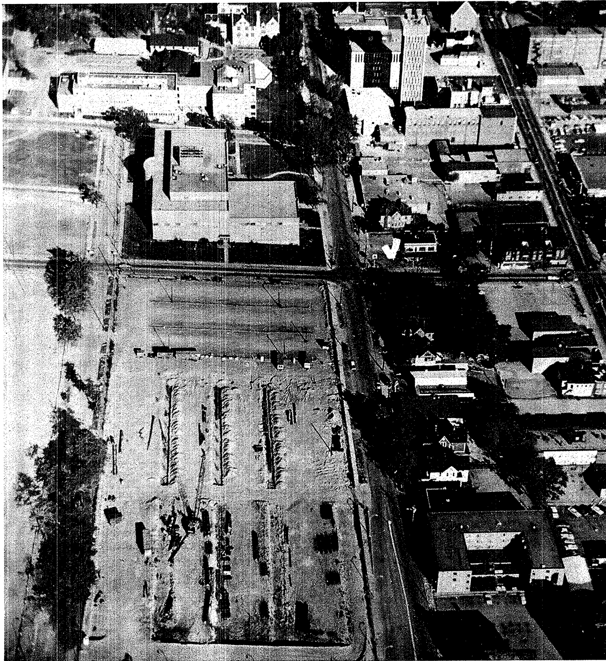
THE PARKING DECKS THAT MIGHT BE — Construction on the parking decks in the student parking lot off Arlington is not now expected to be completed until after fall quarter has begun. The parking decks construction site can be seen in the bottom left of this aerial photo.
