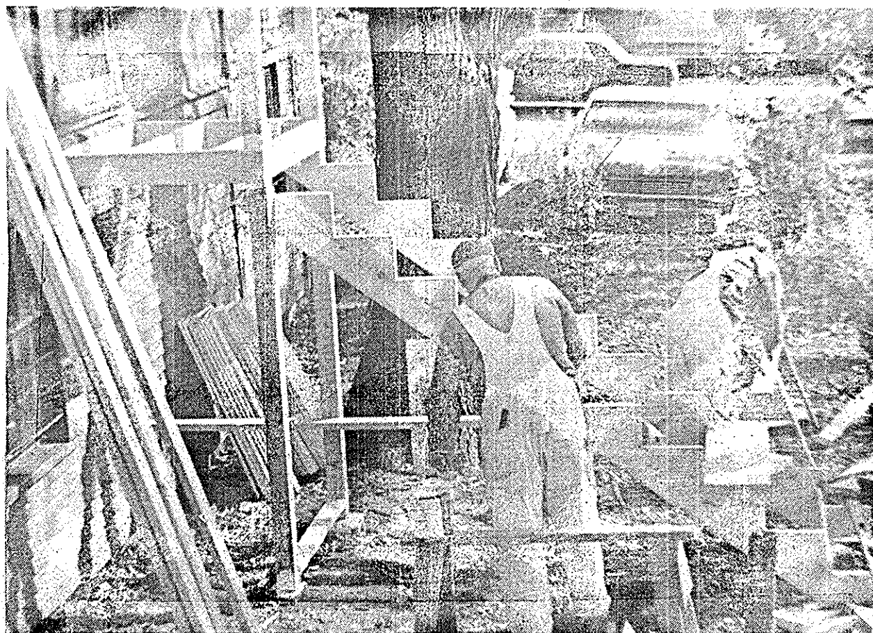
Carpenters hard at work on the new stairs for the NEON office
