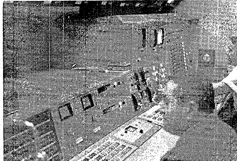
Technicians monitor similar equipment to what we expect at YSU.
