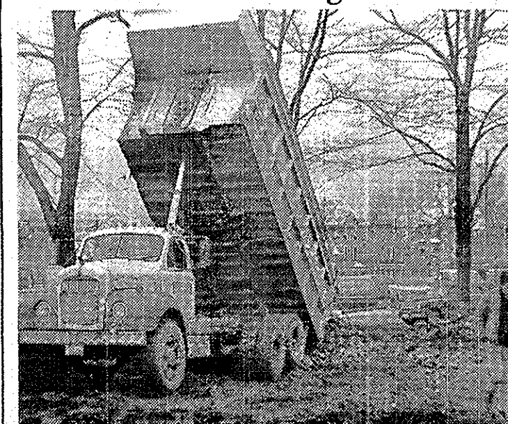
Refuse resulting from the demolition of houses in Phase II of the Urban Renewal Project is trucked away.
