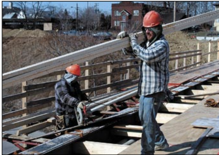
Construction worker Michael Hedrick carries lumber across the Fifth Avenue bridge over Madison Avenue Expressway. Six bridges on the university's northern fringes are being rehabilitated as part of a $7.5 million project to enhance the major entrances to the campus.
