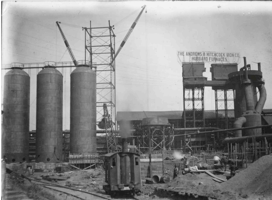
Figure 3-4: This 1910 view shows the construction of the new No. 1 furnace along with the older, hand-fed No. 2 furnace at right. The dust collector shown on the No. 2 furnace acted only as a primary gas cleaning facility, as a gas washer to more thoroughly clean the waste gas was not installed on that particular stack until 1915. The covered stock house for the furnaces can be seen directly behind the elevator shafts.
