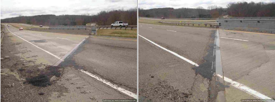
Fig. 3.4 – Pictures of bumps at Bridge No. COL 30 2670.
