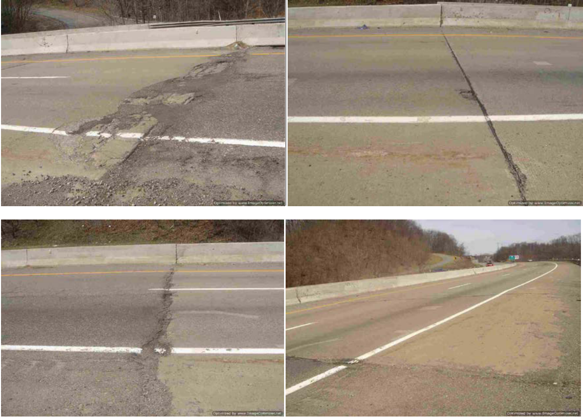
Fig. 3.5 – Pictures of bumps at Bridge No. COL 30 3182.
