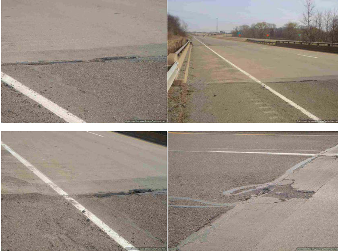
Fig. 3.3 – Pictures of bumps at Bridge No. COL 11 2L.
