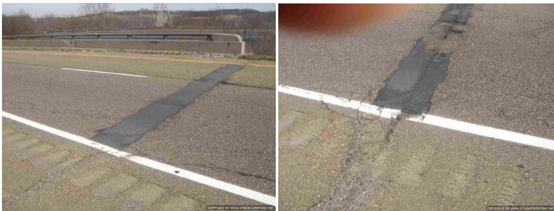
Fig. 3.1 – Pictures of bumps at Bridge No. COL 30 2578.
