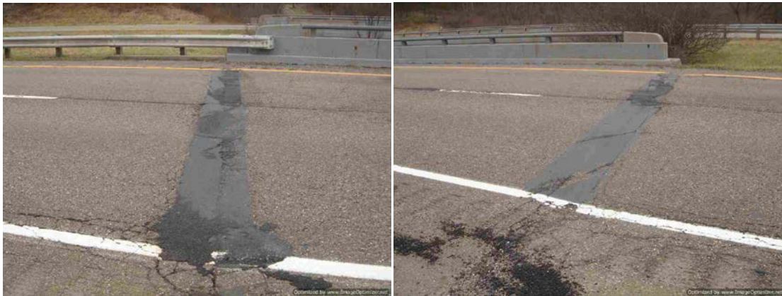
Fig. 3.2 – Pictures of bumps at Bridge No. COL 30 2667.
