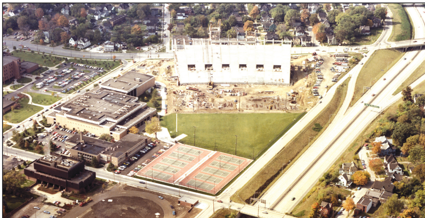
The preliminary construction phase what of would end up as Stambaugh Stadium in 1982. File photo courtesy of Maag Library.
