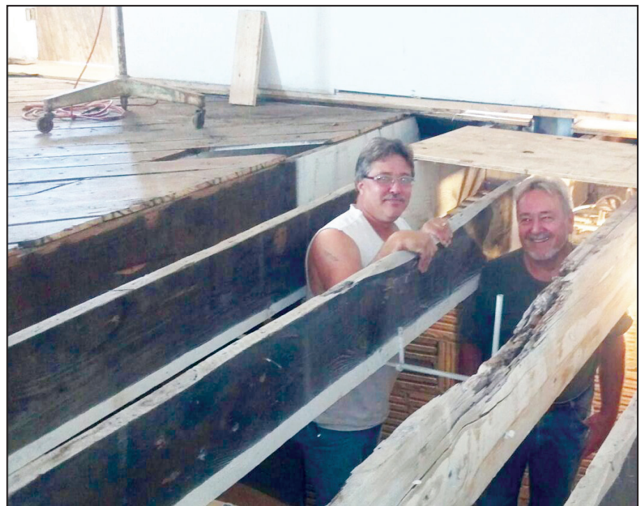
Terry Fusco (left) and Vince Trinckes (right) are just two of the many people from Common Wealth Inc. who have worked on the construction of the Elm Street Cafe that is anticipated to open in spring 2014. Photo courtesy of Christina Perry.
