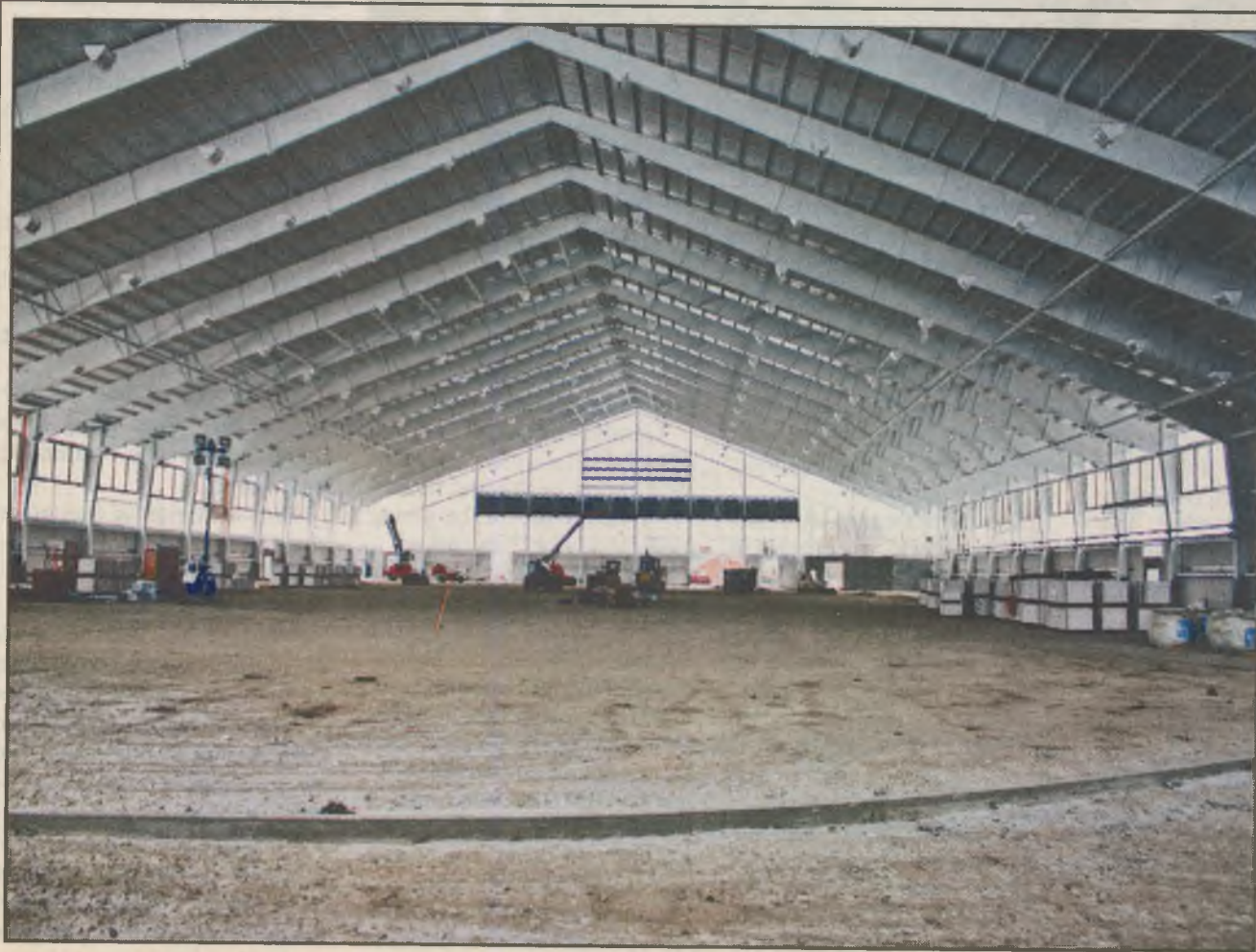
Several setbacks in the the construction of the Watson and Tressel Training Site, shown above, have prevented adherence to either of its completion dates. Hively Construction Superintendent Rodger Shuback, pictured below, said those involved with the project plan to meet Tuesday and discuss when the WATTS will be finished. Photo above by Nick Young/The Jambar, photo below by Doug Livingston/The Jambar.
