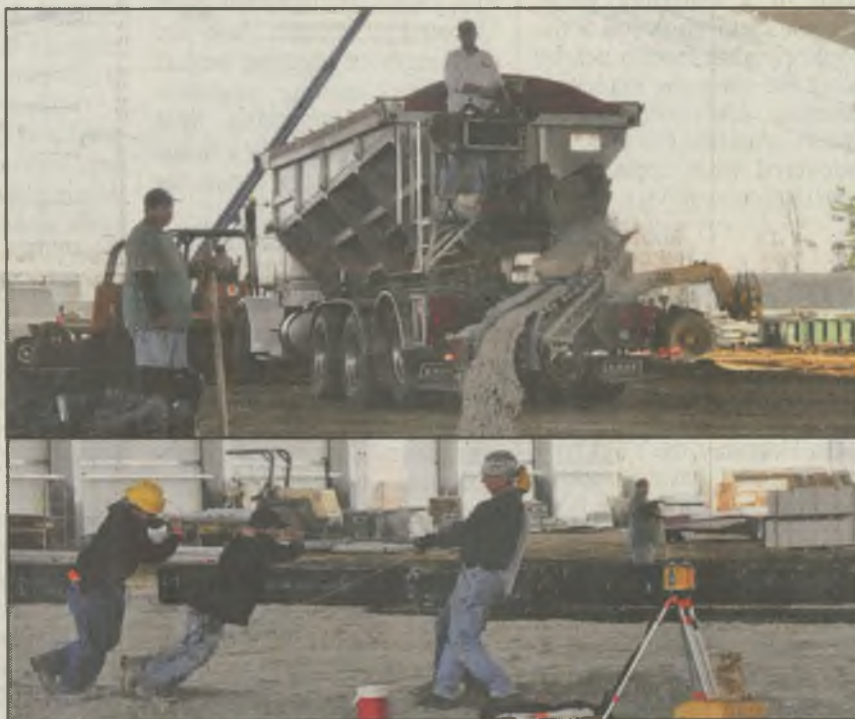
Workers continue construction on the WATTS, which is now slated to open in February. Weather has delayed completion of the project by several months and is forcing construction crews to continue work into the winter.
