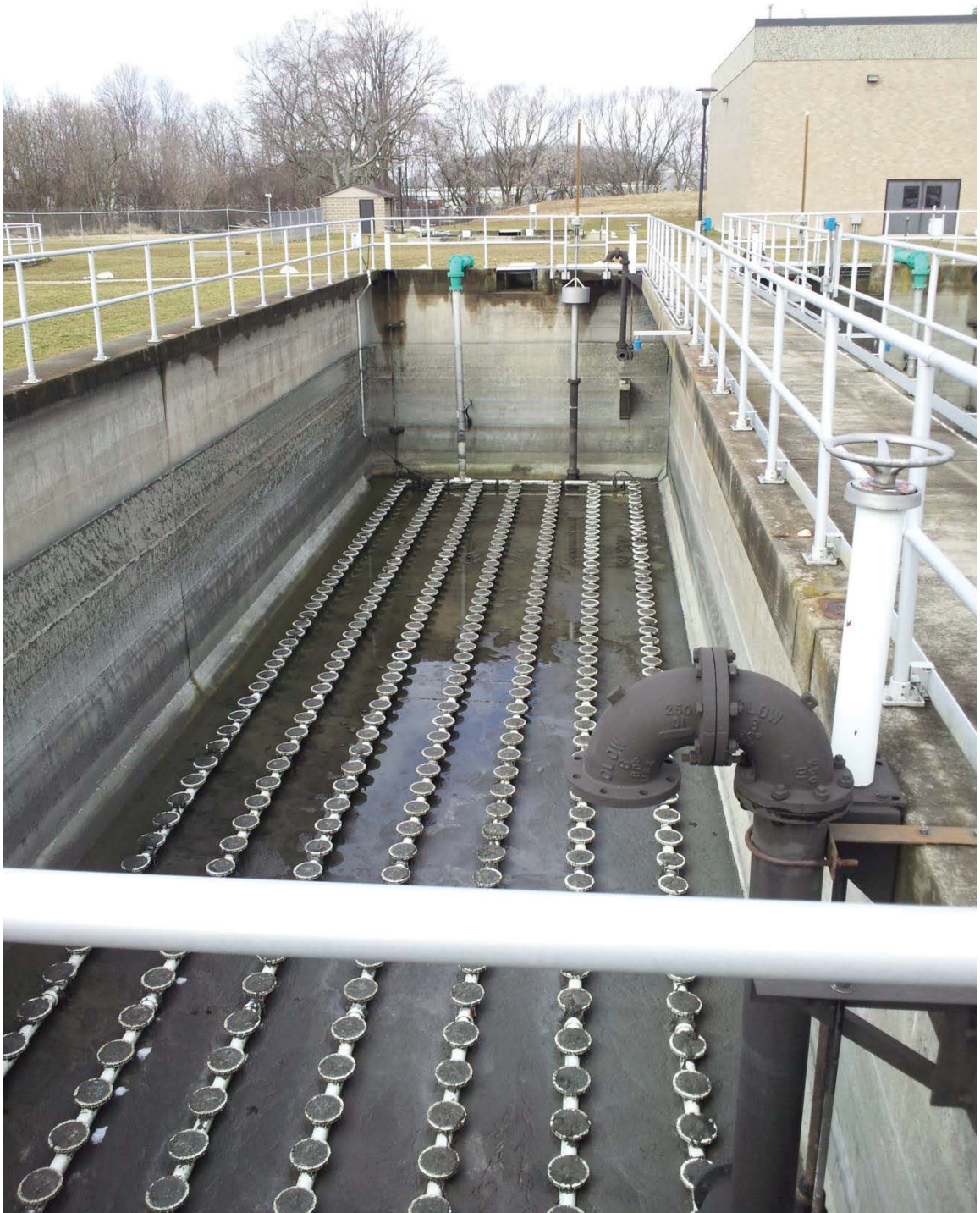
Figure C.1: Aerobic digesters at Columbiana WWTP
