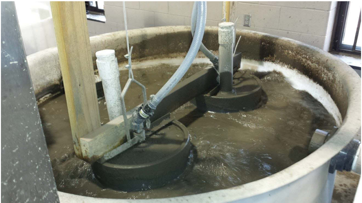
Figure C.14: Process tank 3 in steady-state
