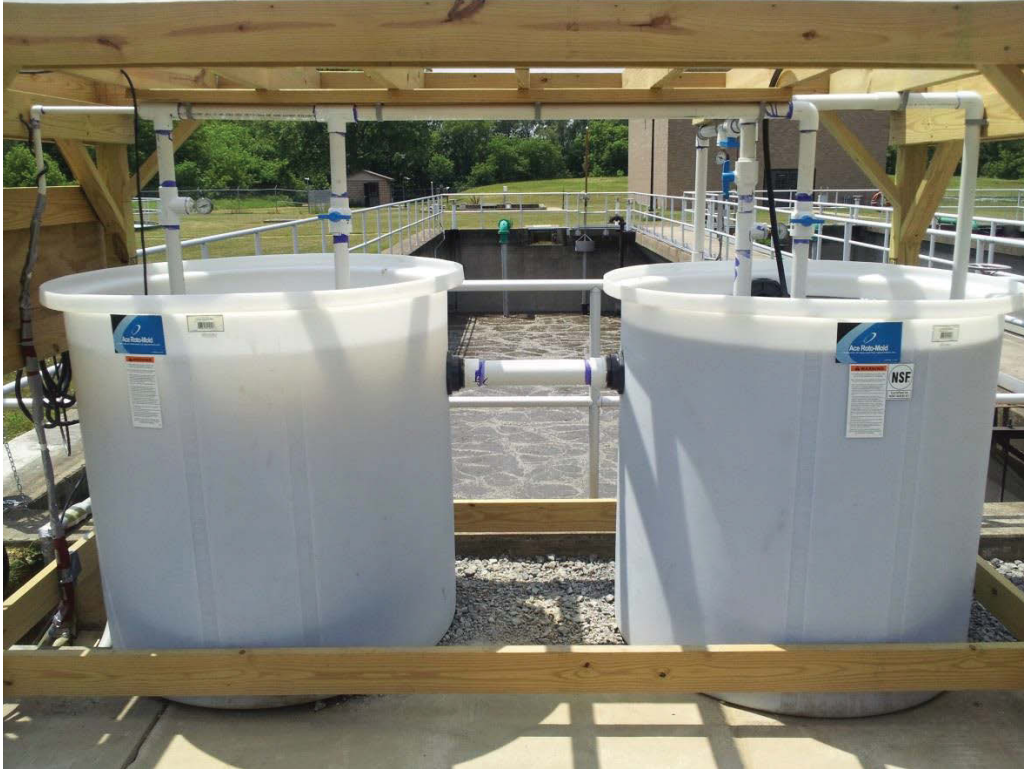
Figure C.2: Primary and secondary holding tanks
