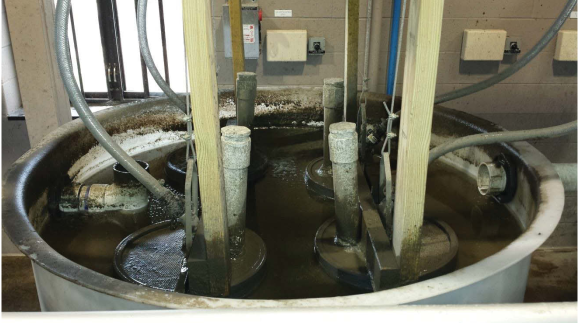
Figure C.13: Process tank 2 in steady-state
