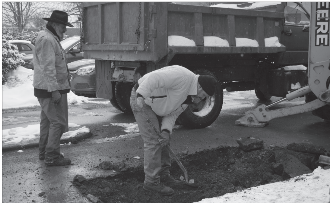
A water main broke Monday evening next to Fedor Hall. Maintenance crews worked to repair the break, though were not able to stop the basement of Fedor from experiencing residual flooding.
