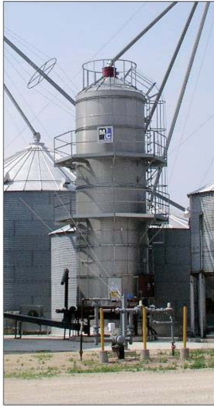
Figure 1.2-1: Typical Vertical Cross-Flow Grain Dryer (Wehrspann, 1998)
