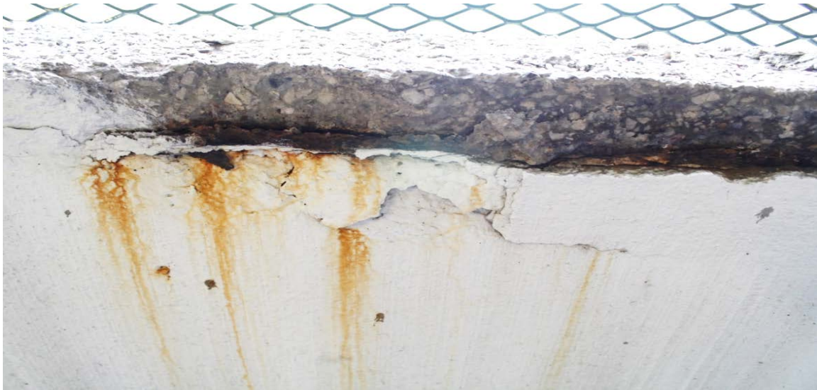
Figure 3-5: Corrosion observed on the barrier wall in Level 1-D.
