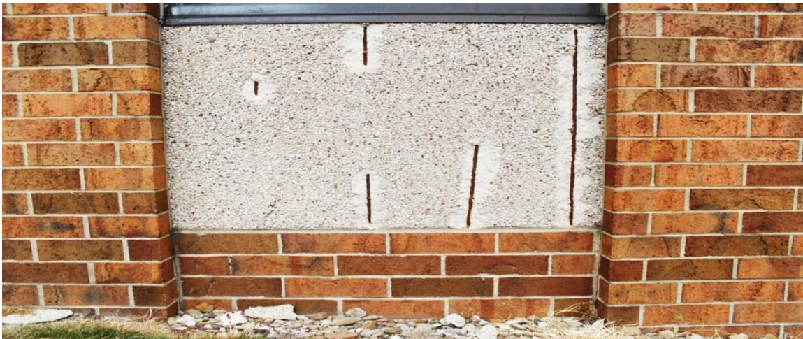
Figure 3-6: Inadequate concrete cover seen on the outside of the exterior walls.
