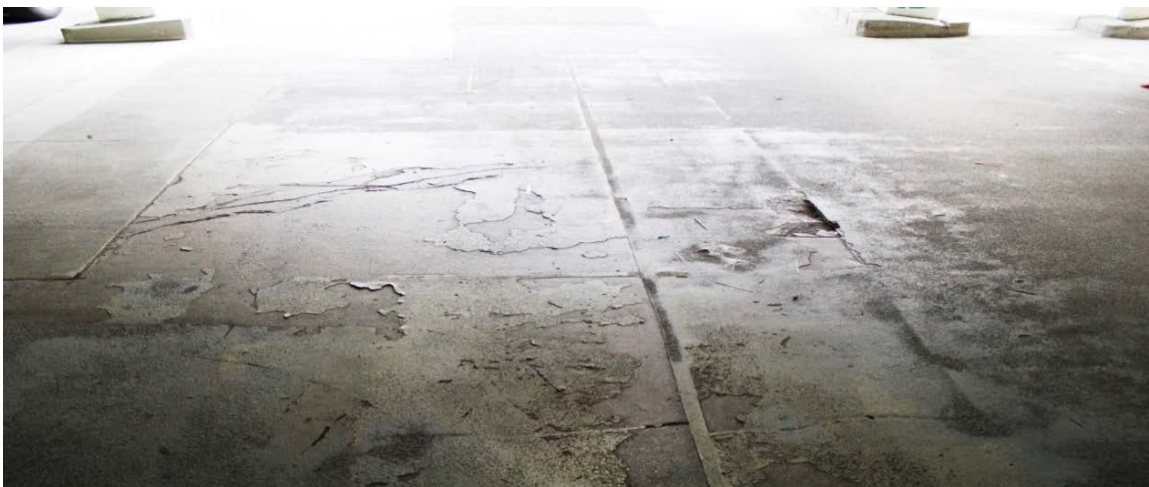
Figure 3-8: Wear and tear caused from tires of the vehicles.
