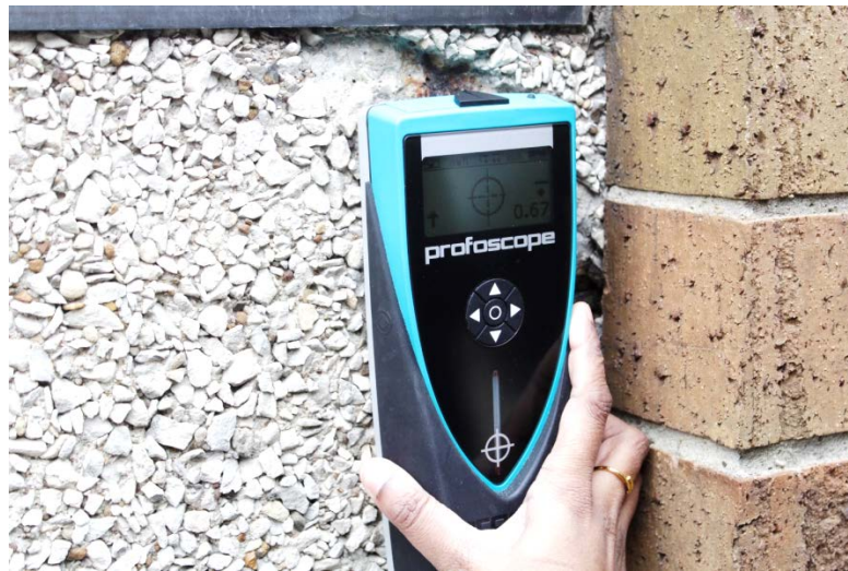
Figure 4-3: The Profoscope being used to determine the depth of concrete clear cover on the wall.
