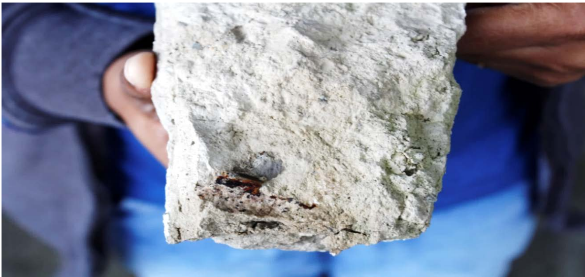
Figure 3-3: Presence of carbonation detected as the concrete turns colorless.
