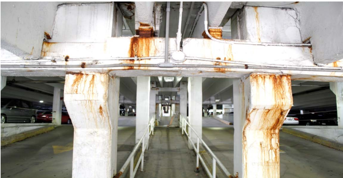
Figure 4-1: Corrosion stains on the columns at Lincoln Parking Deck.
