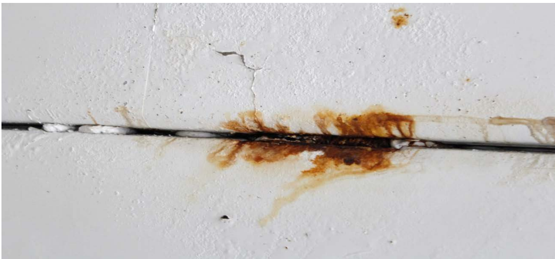
Figure 3-2: Corrosion due to chloride ingress at the joint of two double T-beams.
