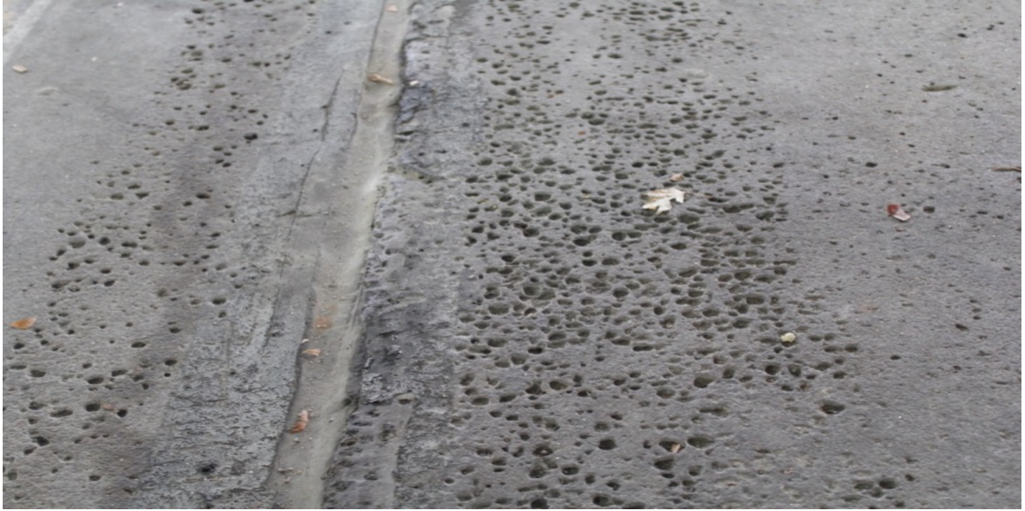
Figure 3-9: Bug holes found on the slabs.
