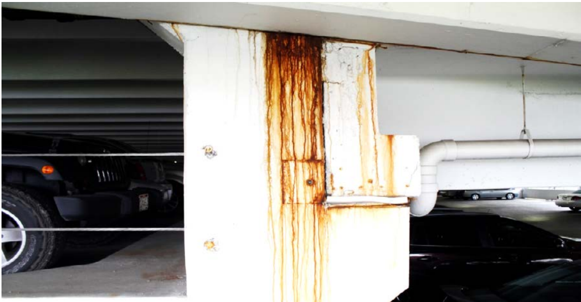
Figure 3-7: Corrosion stains caused due to water leakage.
