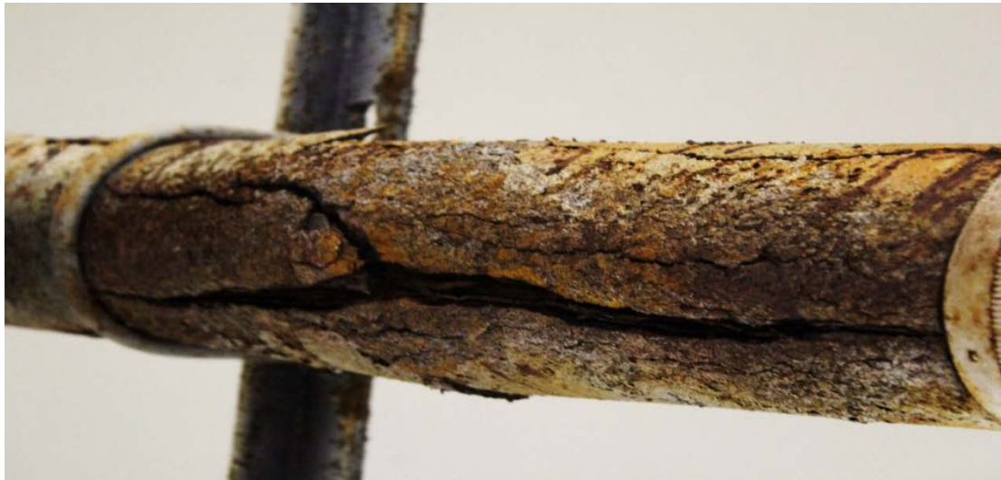
Figure 2-4: Uniform corrosion on the pipes in the Lincoln Parking Deck.
