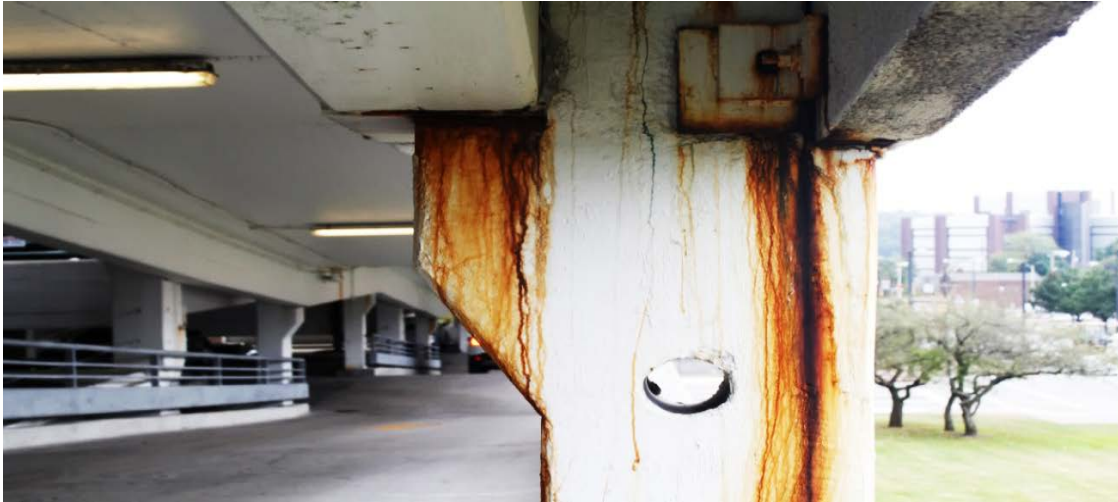
Figure 2-5: Dissimilar corrosion between deck metal plates and bolts in the Lincoln Parking Deck.
