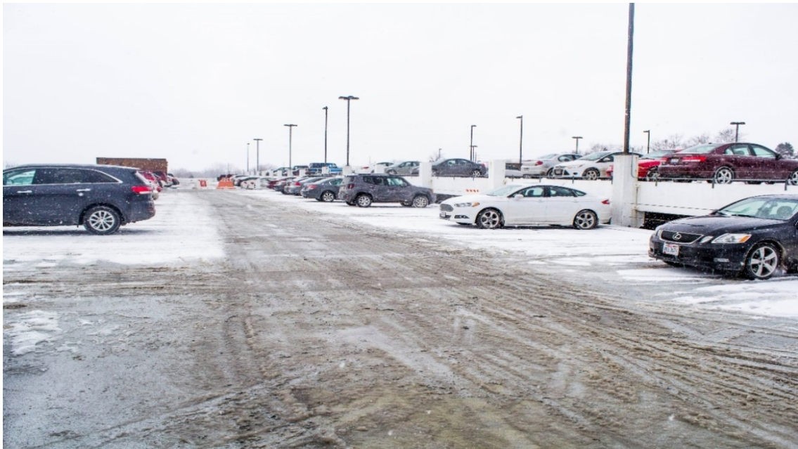
Figure 3-1: Roof of the Lincoln Parking Deck filled with slushy snow.
