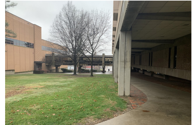
The roof will be replaced on the bridge connecting Cushwa Hall and Moser Hall. Photo by Jordan Boitnott/Jambar Contributor
