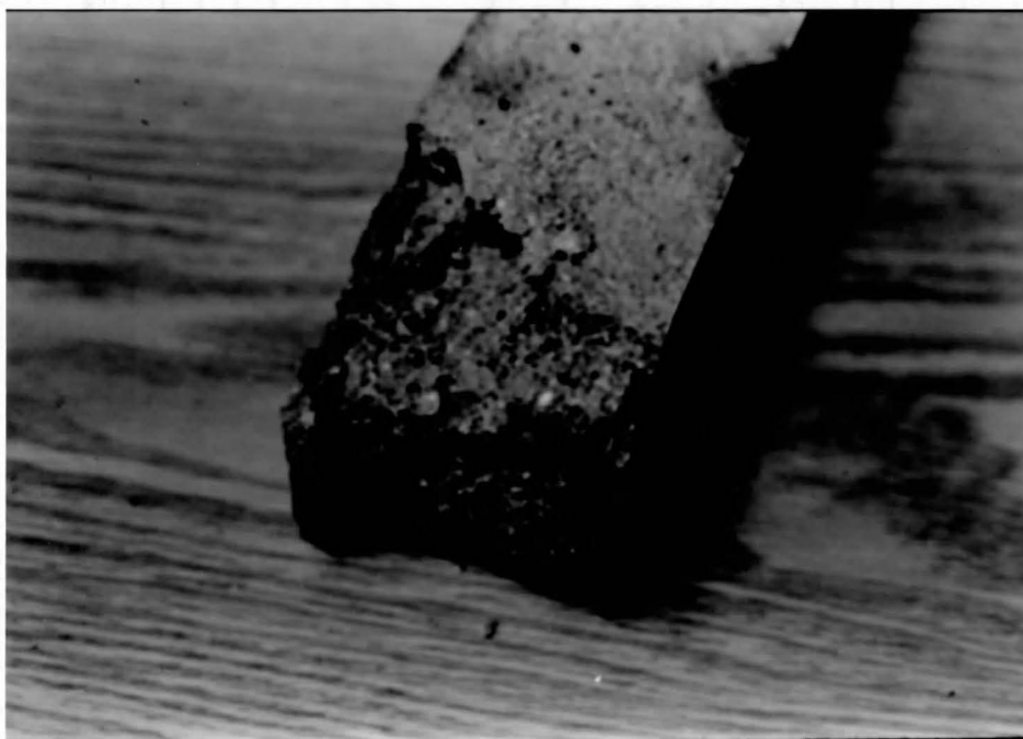
FIGURE 6.7 SPALLING OF LINSEED OIL ON P2 (NOTE LAYERED EFFECT)
