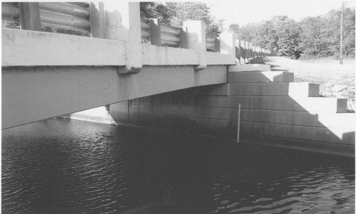
Figure A-2 Photograph of Gauging Station at Yellow Creek near Lake Evans (Site #3).
