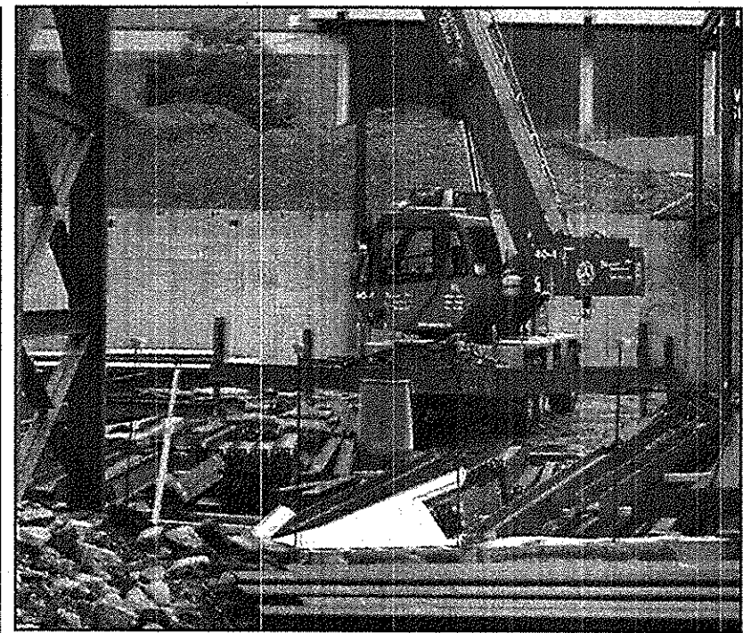
Construction continues on the Andrews Student Health and Wellness Center on the west side of campus.
