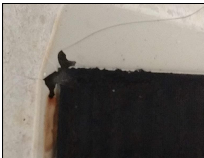
Figure 5.20: Closeup of the chip/crack in Cell #5
