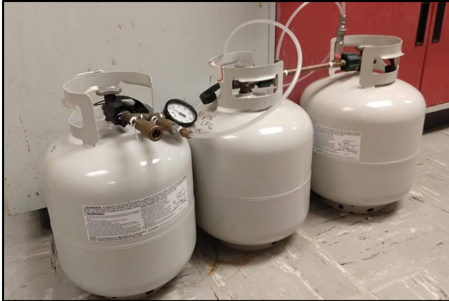
Figure 2.9: Propane cylinders connected with gas tubing contain landfill gas pressurized to 40 psi.
