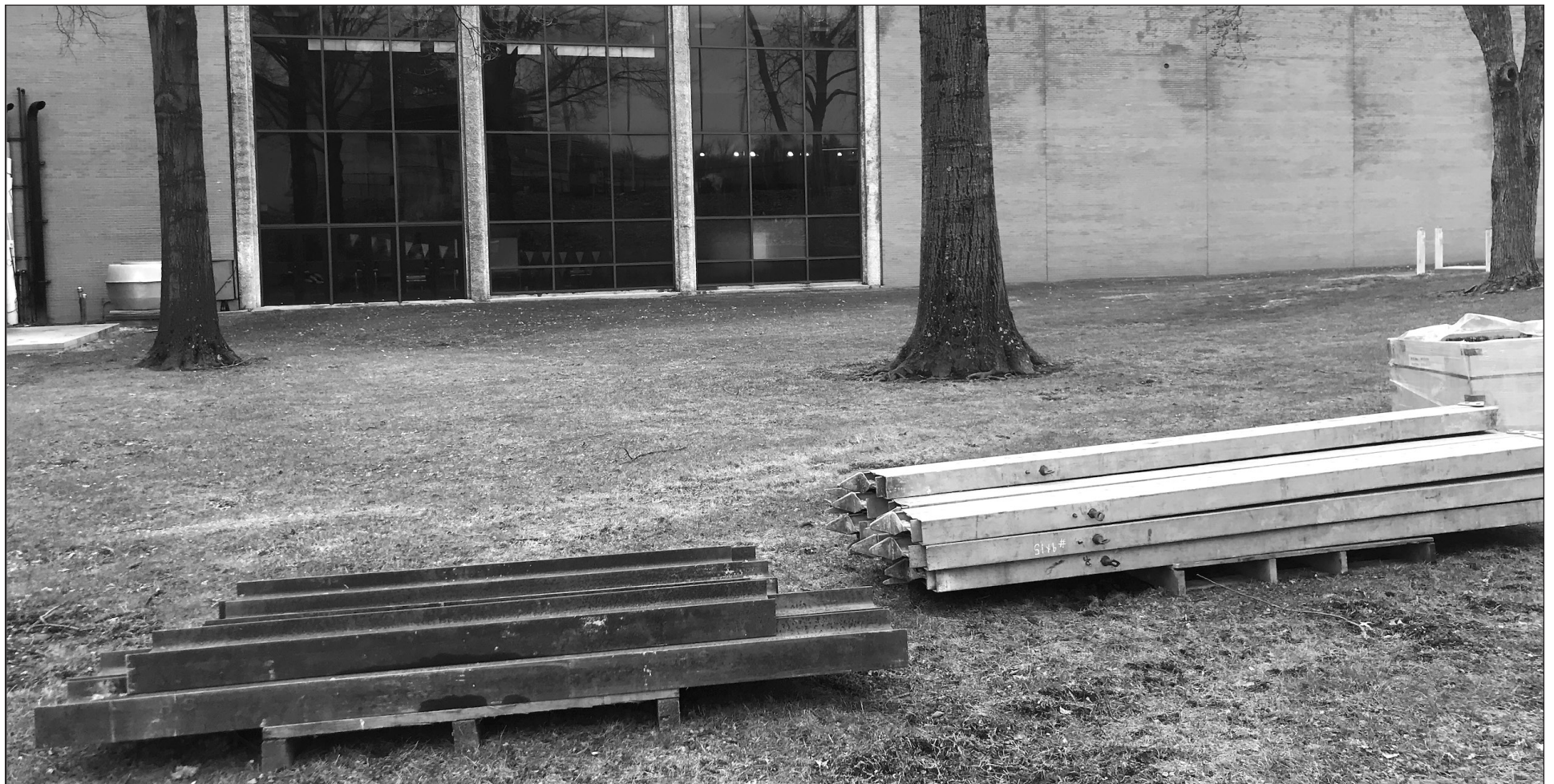
The moisture from the pool in Beeghly Center has worn down the building's exterior.
