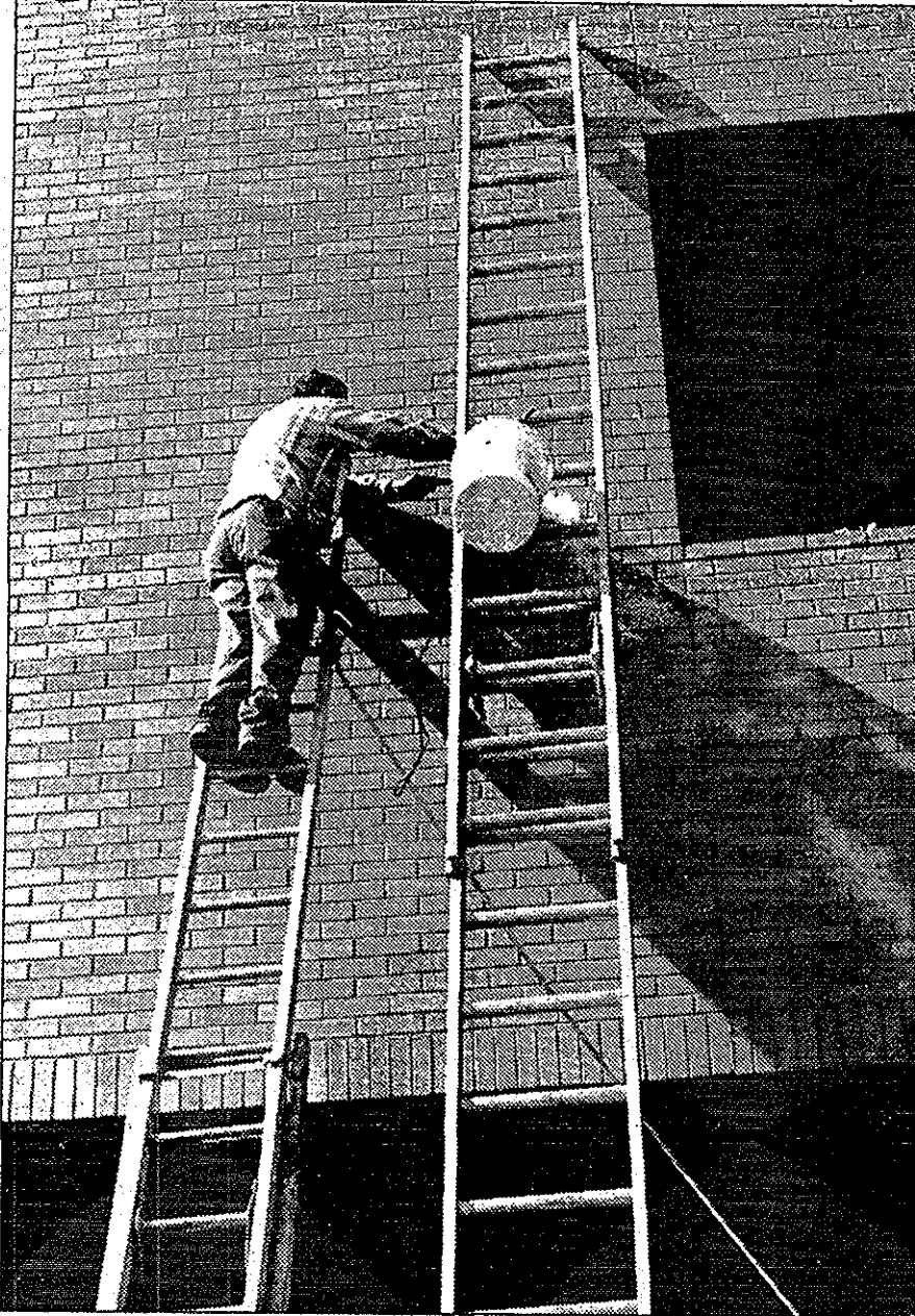
Extensive improvements continue across campus. This YSU worker skillfully balances on a ladder while cleaning the many bricks in DeBartolo Hall.
