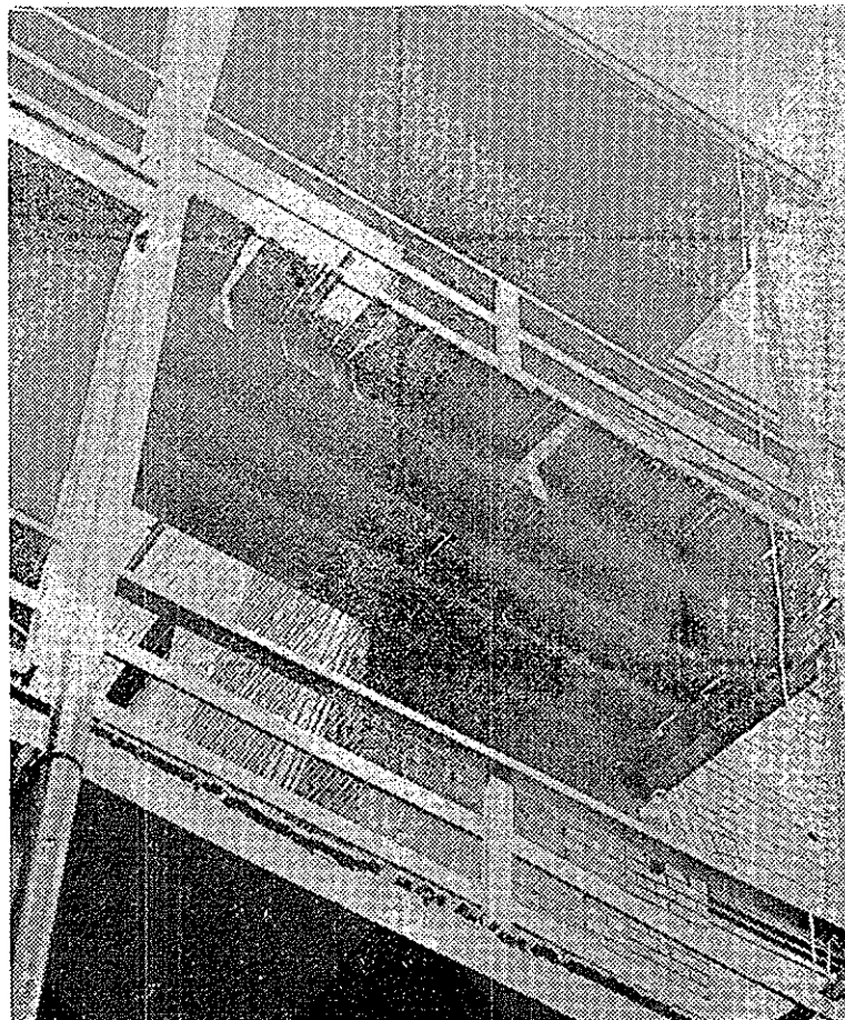
The rotting fire escape at the Lincoln Hotel.
