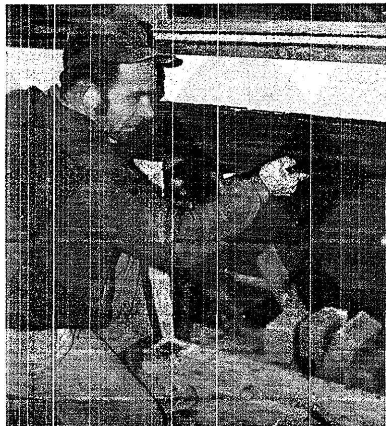
Paul Hines, construction worker for the Kreidler Construction Company, prepares Tod Hall for installation of air conditioning.
