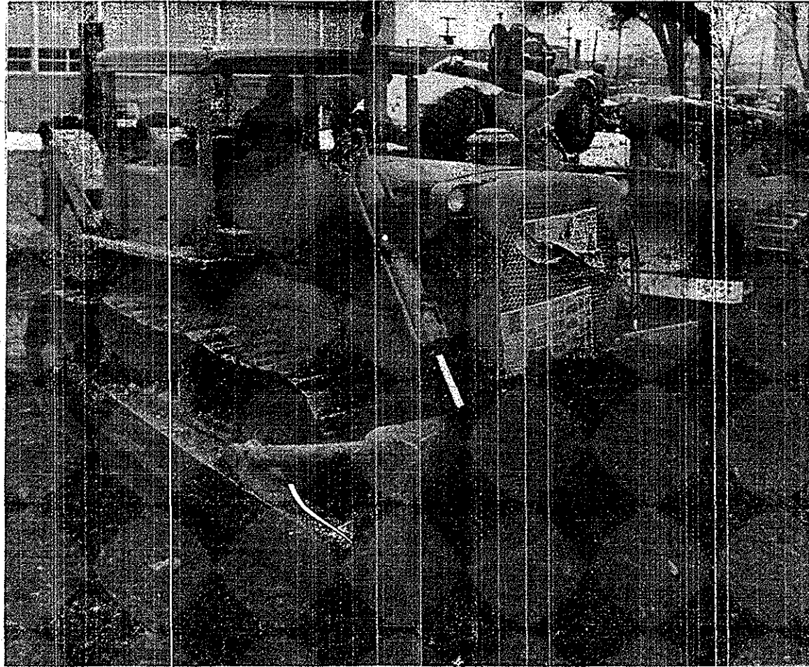
Excavation continues on the $5 million Beeghly Physical Education Center. Though frozen ground has hampered the digging, expected warming trends should offer encouragement.
