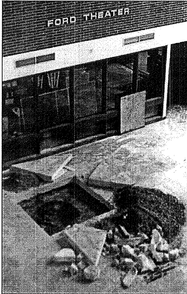
BUILDING A BETTER BLISS: Construction is underway in front of Bliss Hall's Ford Theater. Bliss Hall will be under construction until April 1999.
