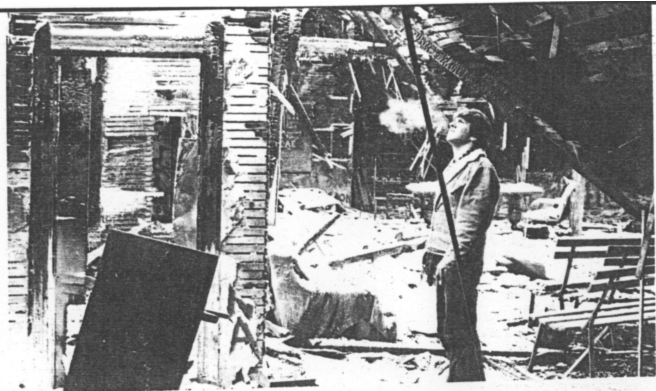
EXTENSIVE DAMAGE — A Sigma Alpha Epsilon fraternity member surveys fire damage to a room on the second floor of the fraternity house on Pennsylvania Avenue. (Photo by Bill Oberman)
