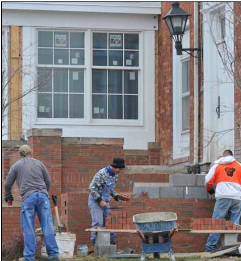
Construction workers continue improvements on Coffelt Hall on University Plaza, the new home to the School of Graduate Studies and Research. It is one of a handful of construction projects on campus this fall and winter.
