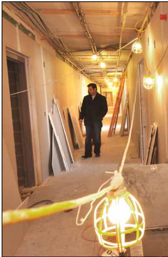
Dominic Marchionda, president of U.S. Campus Suites, walks through a hallway in the Flats at Wick, a 115-bed apartment complex under construction across from the Cafaro House residence hall on the North Side of the YSU campus.
