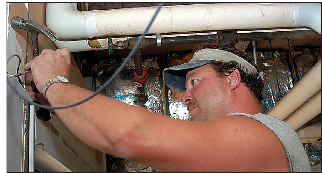
Mike Wolford of Aberdeen Construction in Boardman works in a classroom on the third floor of DeBartolo Hall, where major renovations are underway this summer to 13 classrooms.
